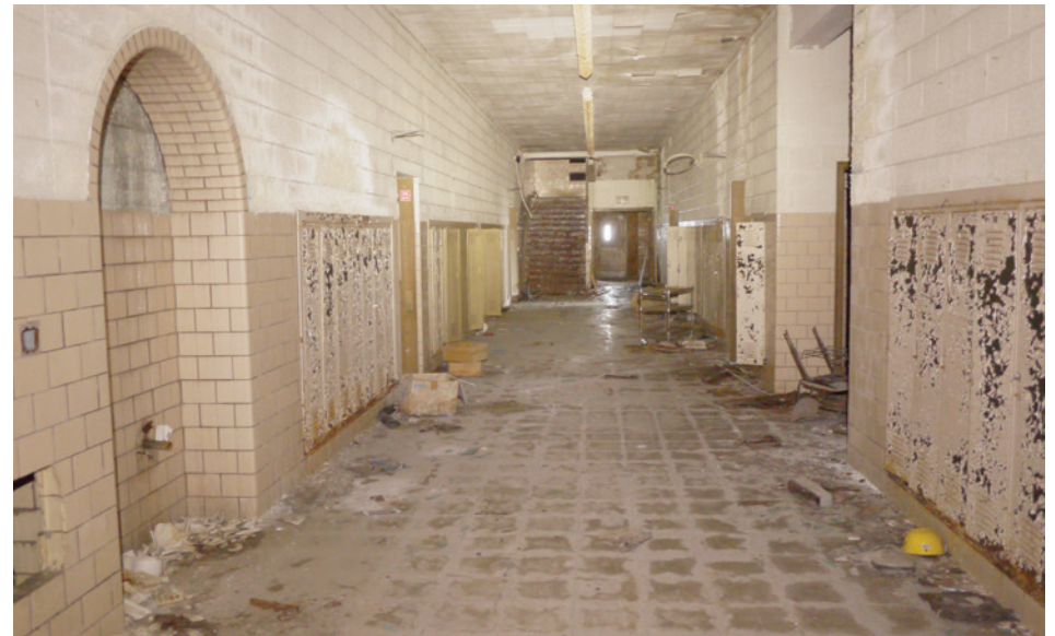
Interiors are simple and sturdy masonry construction, with glazed block accents. Arched alcoves once housed drinking fountains, which have been taken. The corridors do not receive much natural light; the only sources are narrow slit windows in the stairwells at the ends of each corridor.
