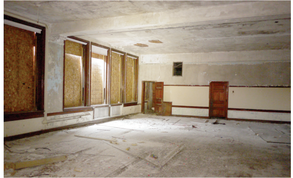
The kindergarten windows. Finishes in classroom areas were in generally good condition.
