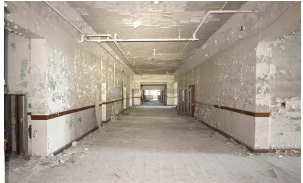
The main corridors in the original 1912 unit are extremely large, at 17' across and 13' high.
