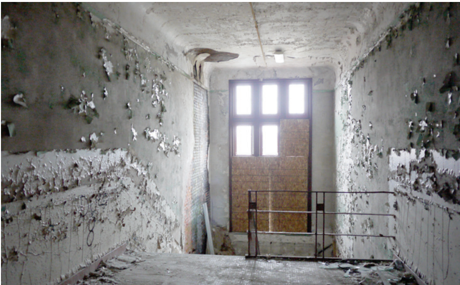
Primary stairwells at either end of the original unit feature 16' high windows that flood the corridor with natural light. Stairwells and corridors feature simple rounded covered ceilings.
