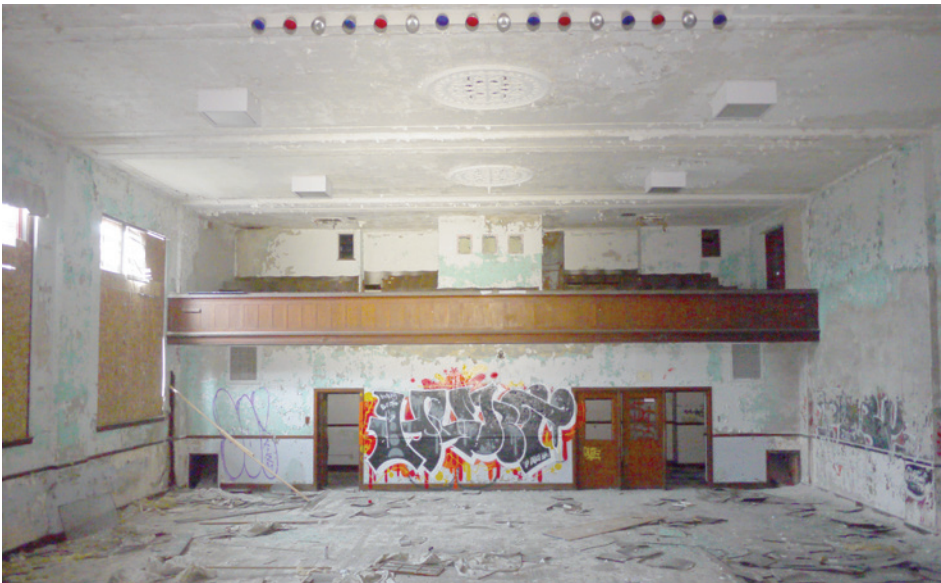
The large auditorium floor and wood-paneled balcony viewed from the high stage. Decorative circular ventilation grilles are visible on the ceiling.
