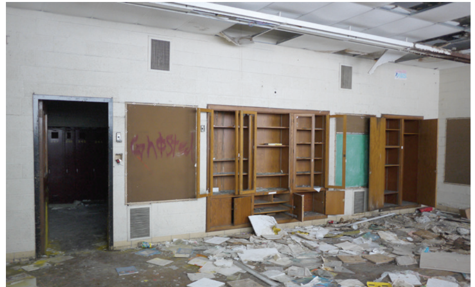
Built-in casework and other finishes in the 1951 classrooms are in good overall condition.
