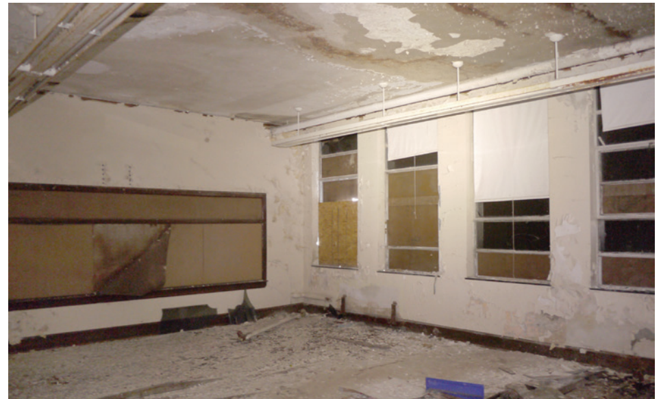
Operable steel windows are generally intact throughout the 1920s classroom wing. These likely date to the 1951 update of the building. Water damage is causing the plaster ceiling to sag.
