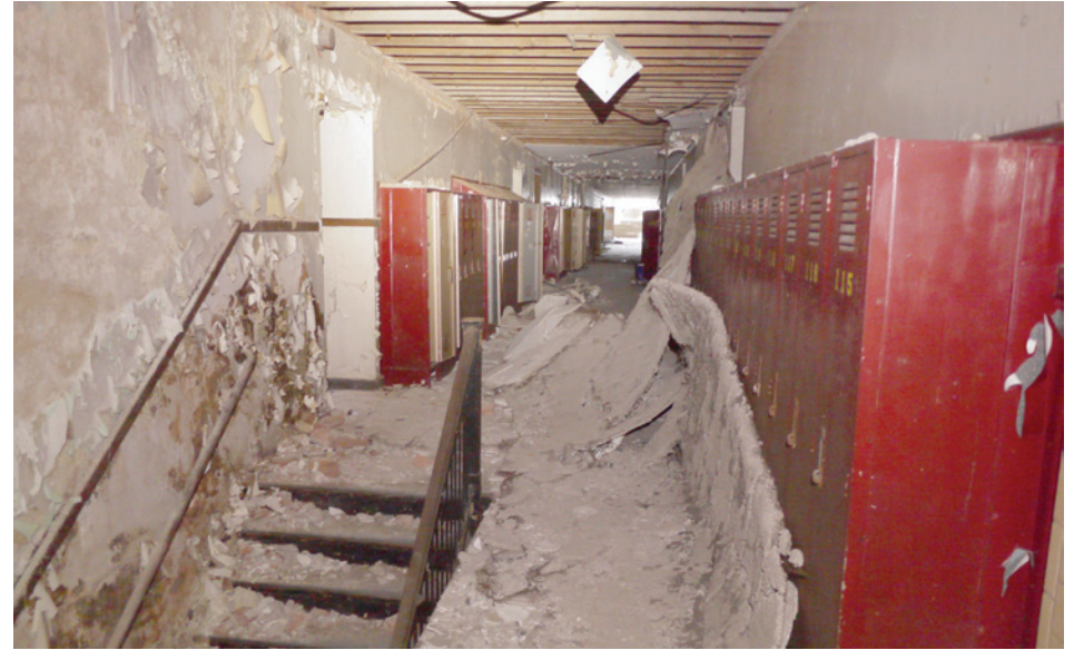
Corridors in the original south unit are 10' wide wall to wall, but feel narrower due to locker banks added later. Water infiltration in the south unit has caused the second floor's plaster ceiling to collapse and has caused widespread water damage in classrooms on both floors.
