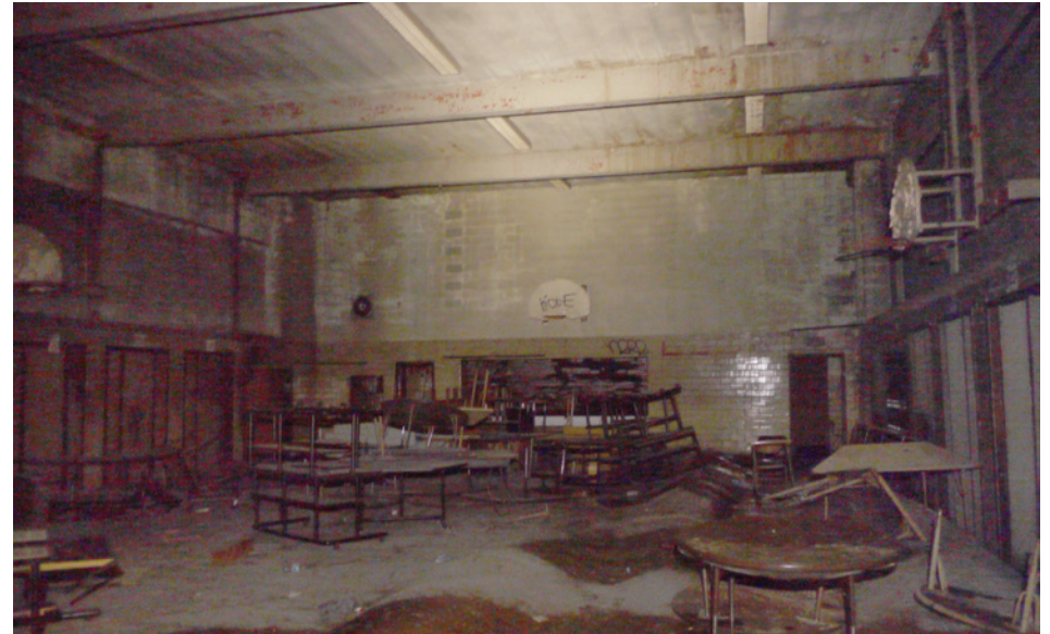
The 1951 gym is a windowless CMU box. Historic floorplans show that there were originally windows on both the north and south walls (presumably glass block matching the classroom addition). These windows were filled in with brick and CMU at an unknown time.
