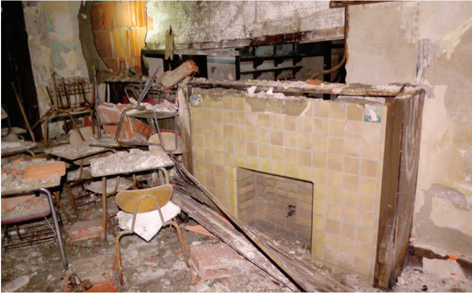
The kindergarten has been heavily damaged by water, fire, and scrapping. Most finishes have been destroyed, but this tile fireplace with prized Pewabic tiles may still be salvaged. Despite the rough appearance, however, the building's structure itself appears to be sound.
